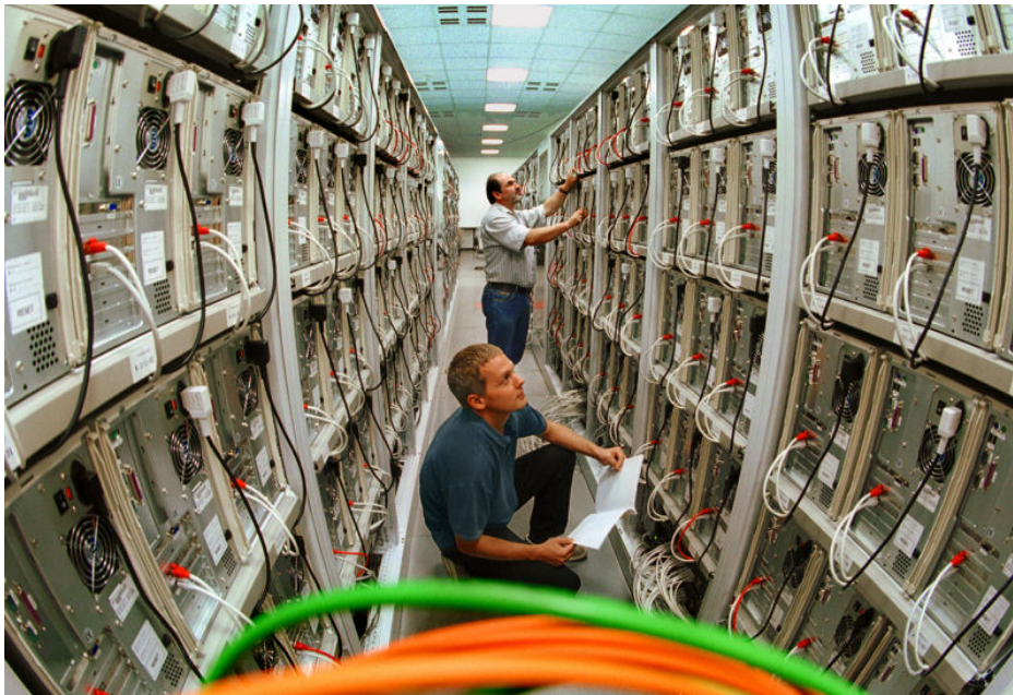
Figure 3.3: Cold aisle between two rows of servers
