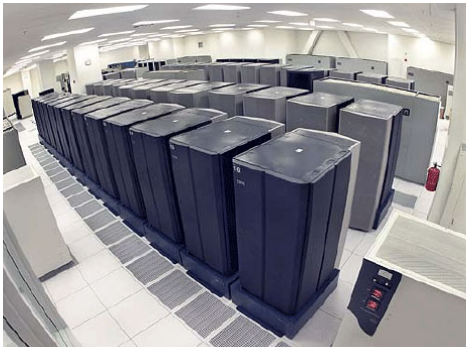
Figure 3.2: A typical server room
