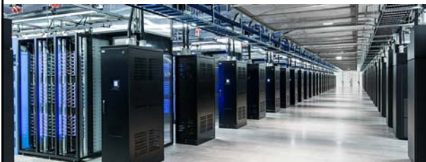
Rack or blade-mounted servers
